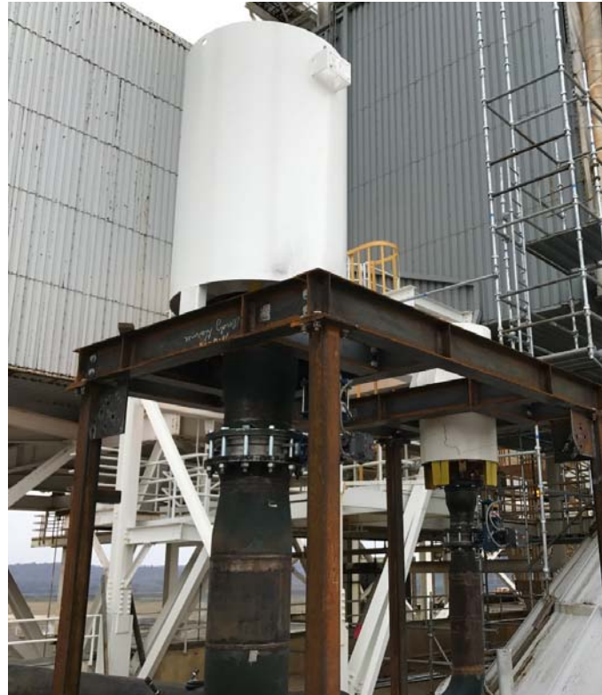
Dual blow-off valves with silencers
